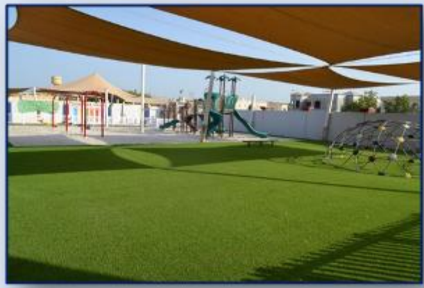
Replacement of turf and shading in KG2 area – for improved safety and comfort
